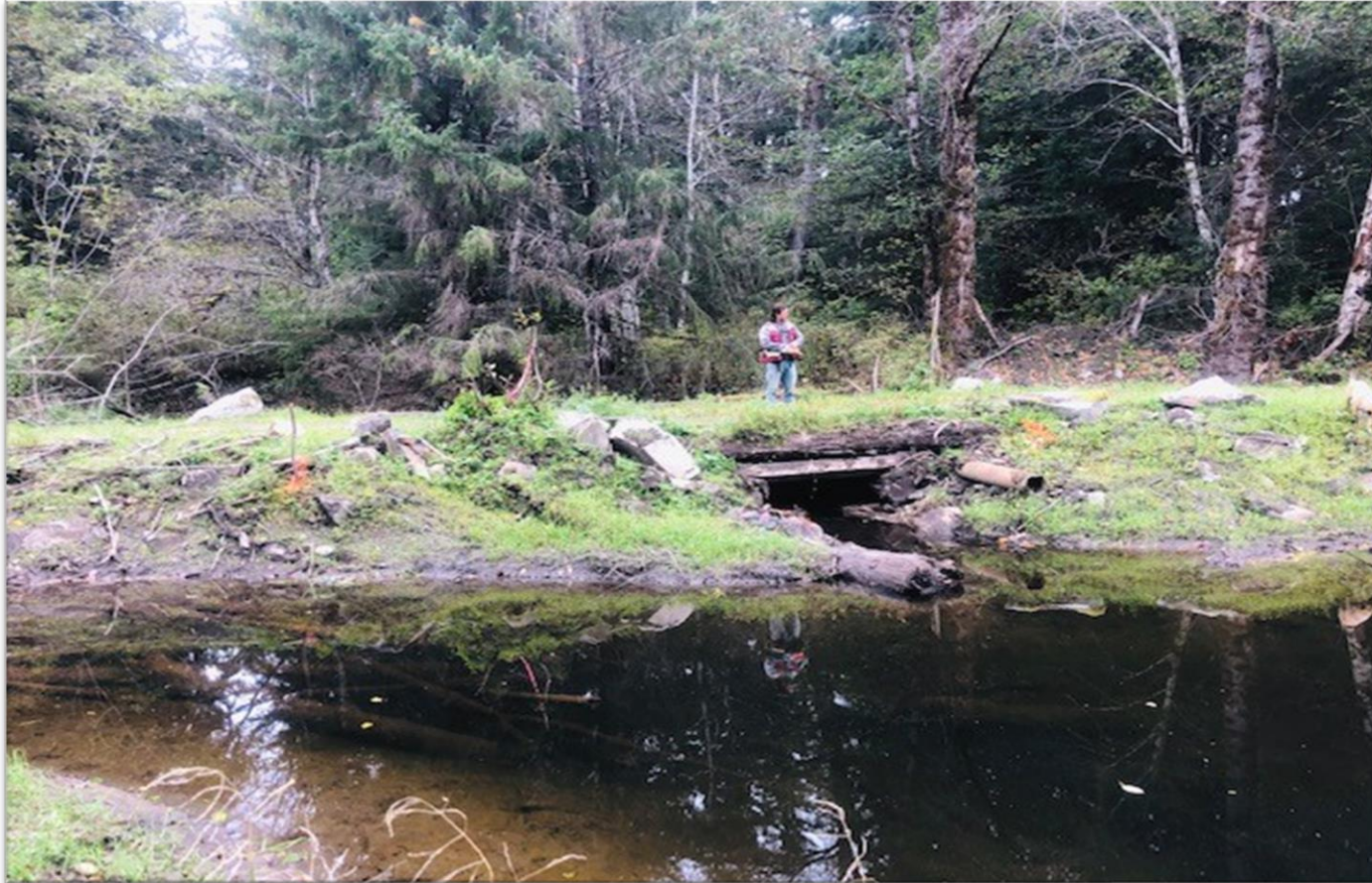
Wood Box Culvert long standing fish passage issue adjacent Nass River Structure confined channel causing flooding, fish stranding and fish mortality
